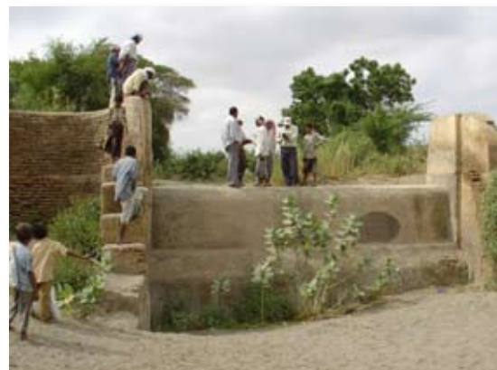
Figure 1 Drop structures to overcome level differences and dissipate energy: note the stepped construction
