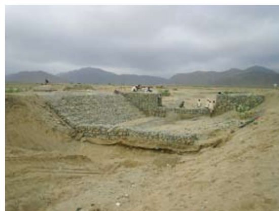
Figure 2 Flow division and channel bed stabilizer: important that apron has sufficient length
