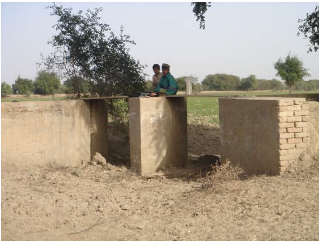
Figure 9 Intake gate with stop-logs
