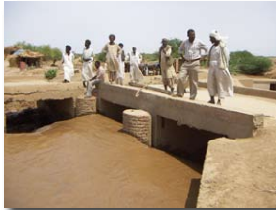
Figure 15 Flow divider at Makala channel, Gash, Sudan.
