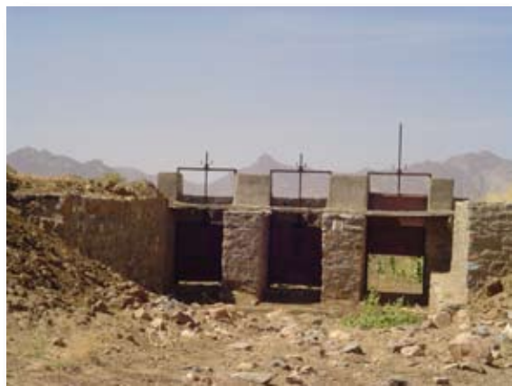
Figure 12 Intakes and sluice gate to improved small system, Alebu (Gash Barka), Eritrea.
